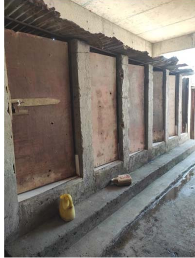
SANITARY FACILITY PROVIDED ON SITE FOR WORKER
